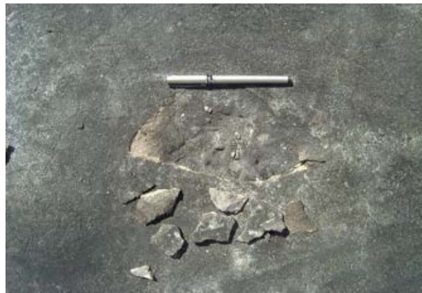
Figure 4 Aggregates are peeled off from the top layer of the concrete on an airbase apron.
