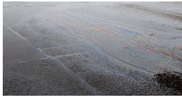
Figure 3. Oils are floating on the run-off water on an apron
